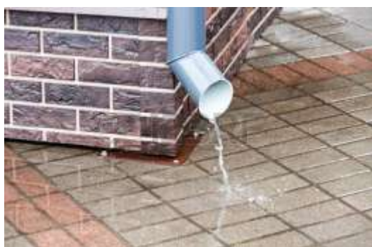
Figure 3: Drainpipe (without filters)
