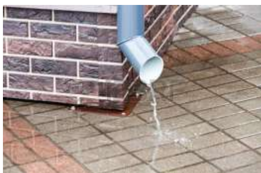
Figure 3: Drainpipe (without filters)
