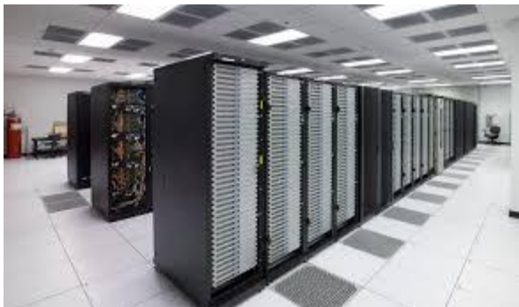
Figure 1: The view of a data center
