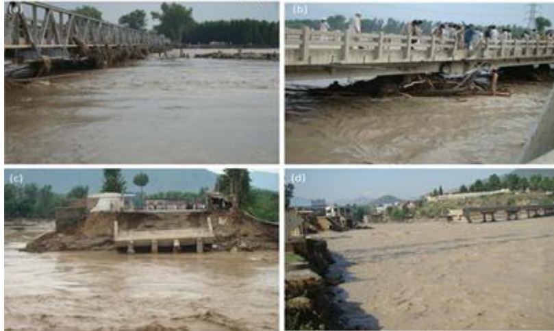
Figure 7: Flood Damage in Indus River Basin at 2010
