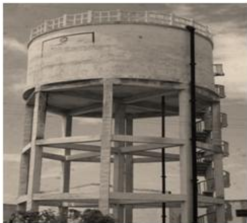
Figure 2: Shows Elevated water tank
