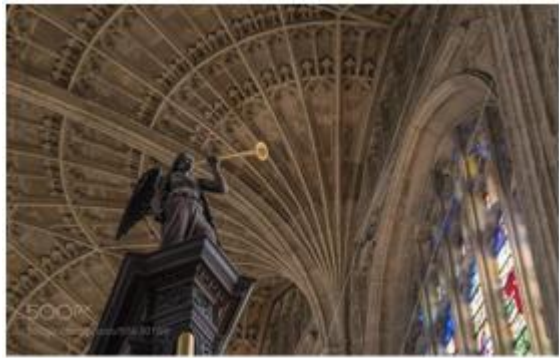
Photo 9: Shows ribs formation in King's College Church van vault roof structure Source: King's-College-Chapel-Cambridge-23486
