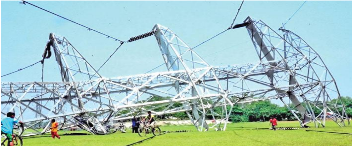
Figure 1: 230KV power transmission tower at Bhairab in Kishoreganj broke down due to tornado
