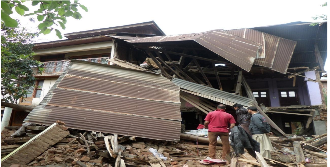
View of damaged house of Muhammad Ashraf Lone at Dal Lake Gagribal, Big Rock boulder is not visible as the roof has coved it
