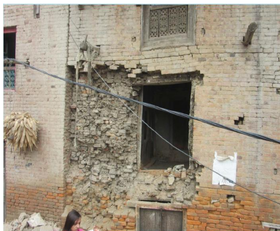
Figure 2: Delamination on masonry building [6]
