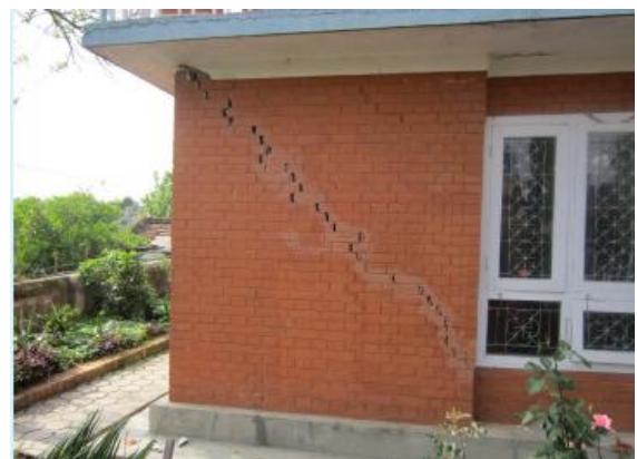
Figure 4: Diagonal Cracks on Masonry wall (NSET, Nepal)[6]
