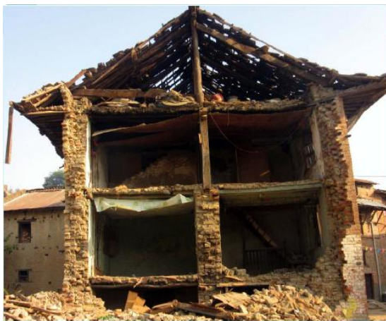
Figure 1: Failure of exterior walls on Masonry building [6]
