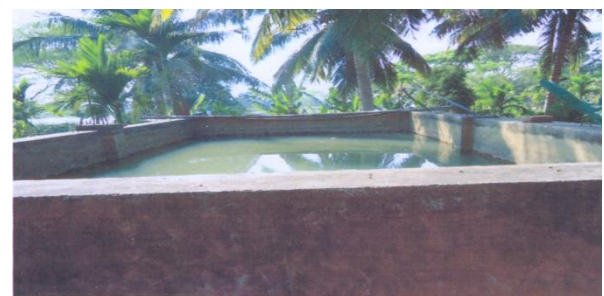
OVER HEAD TANK WITH WATER
