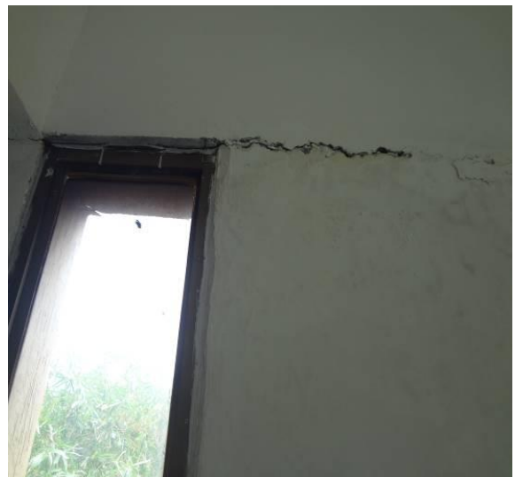
Photograph 11: Beam-wall (Horizontal crack)
