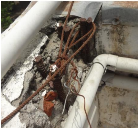
Photograph 3: Open reinforcement and Environmental Effect
