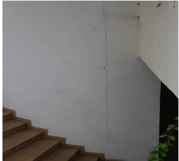
Photograph 10: Beam-wall / Vertical crack (Expansion joint)
