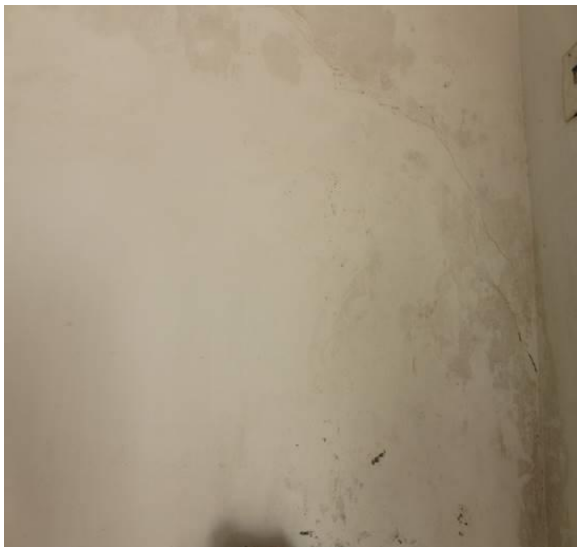
Photograph 8: Near vegetation (Diagonal cracks)
