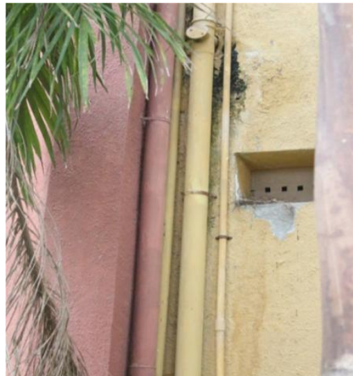
Photograph 5: - Improper/poor drainage pipe
