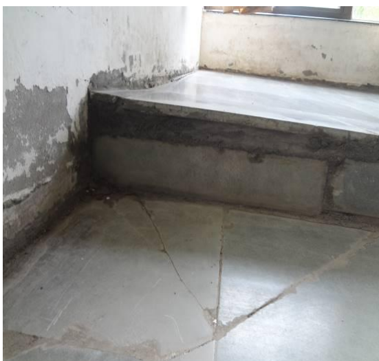
Photograph 9: Flooring/ Improper leveling
