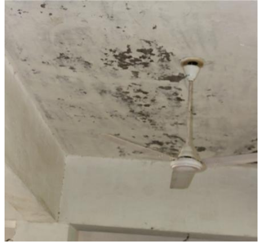
Photograph 4: Leakage and Dampness
