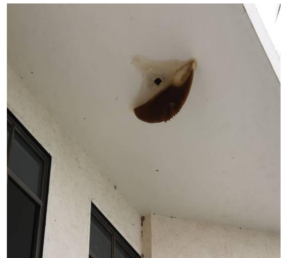
Photograph 12: Lack of maintenance
