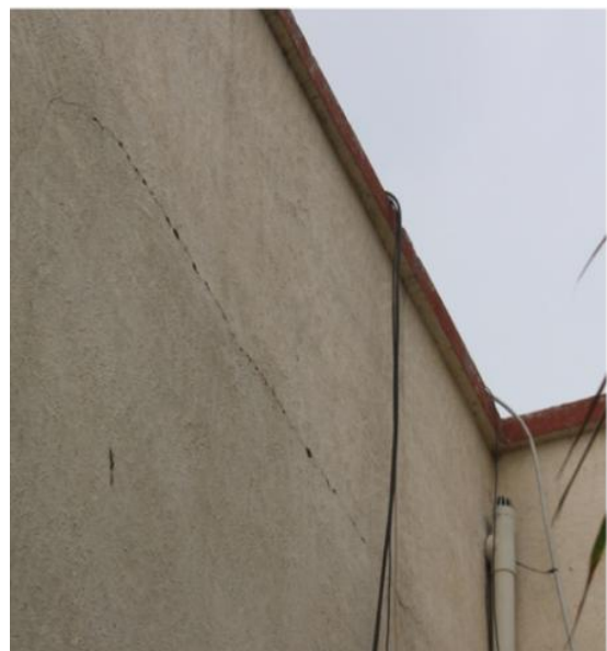
Photograph 6: Horizontal crack due to shrinkage
