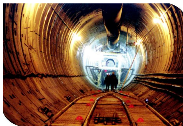
Figure 23: St. Clair river tunnel precast tunnel lining segments.
