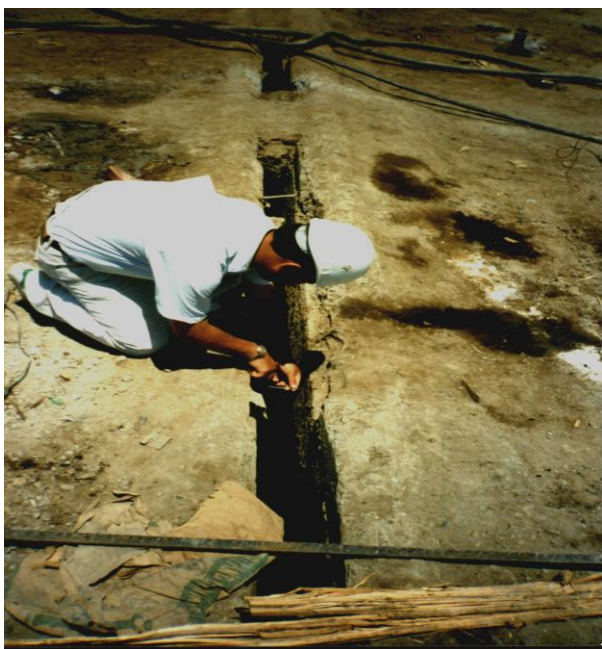
Figure 4: Wide gap due to differential settlement in Damietta bridge
