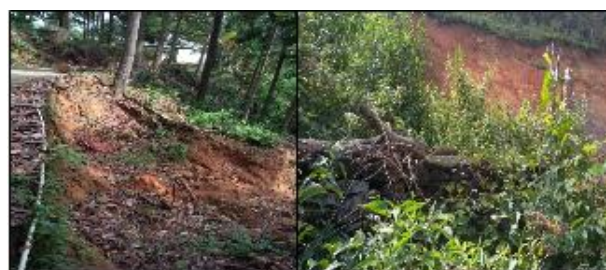
Figure 5: Collapse embankment and Stone bund (Elangapitiya hazard area)
