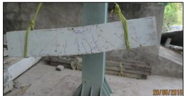
Figure 6.1: Deflected beam and crack patterns
