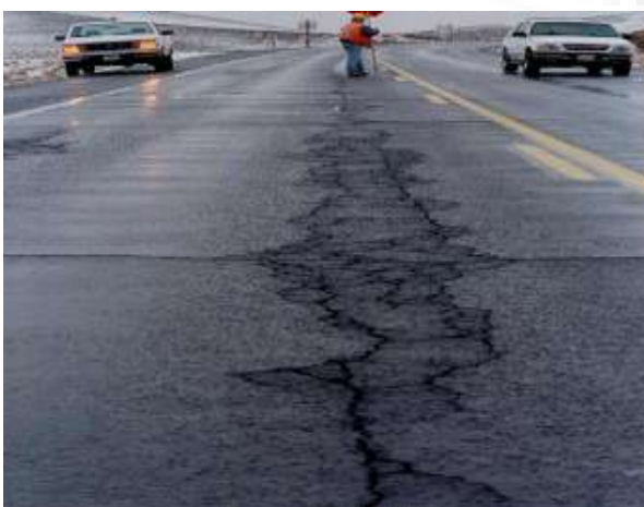
Fatigue: cracking caused by stripping at the bottom HMA
