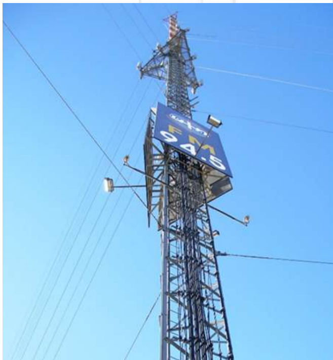
Figure 1: Typical guyed mast
