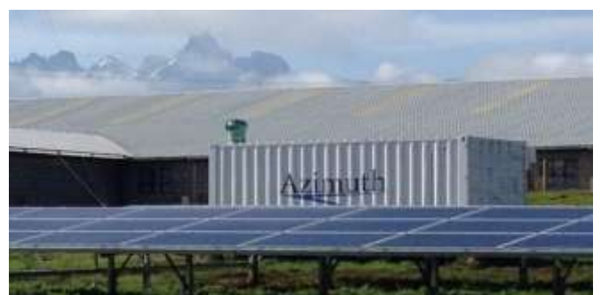
Figure 2: 180kWp solar PV plant at Timafloor Limited Flower farm
