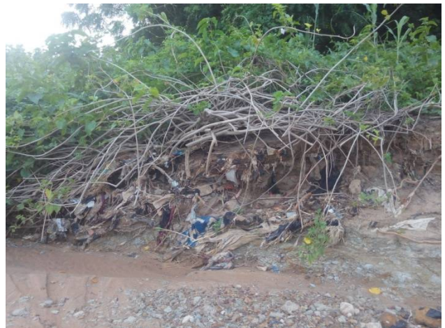
(Plate 5). Gully erosion in Bagadaza
