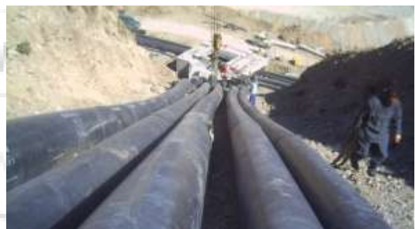
Figure 10(a): Photograph of HDPE Pipes
