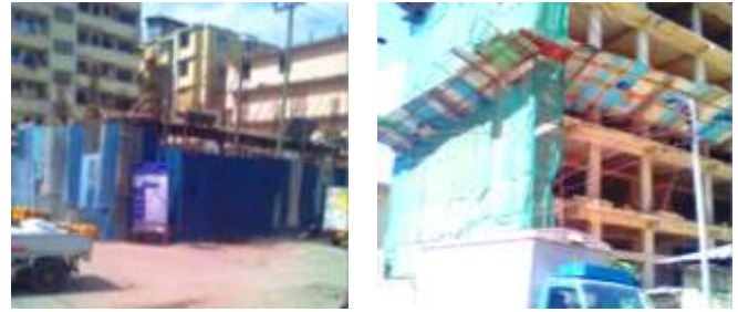
Plate 4.05: (Left) electric transmission lines near the site; and (Right) electric shock hazards due to electrical post near the site, Source: Author,(2017).
