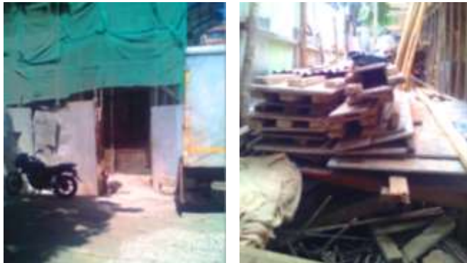
Plate 4.08: (Left) entrance gate of a confined building construction site without health and safety policies in the main entrance; and (Right) inside of a confined site without health and safety policies within the site, Source: Author,(2017).
