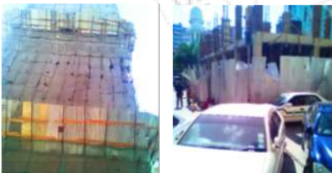
Plate 4.04: (Left) falling hazard at height which has been barricaded; and (Right) hazard working at 2 meters or more above the ground, Source: Author,(2017).
