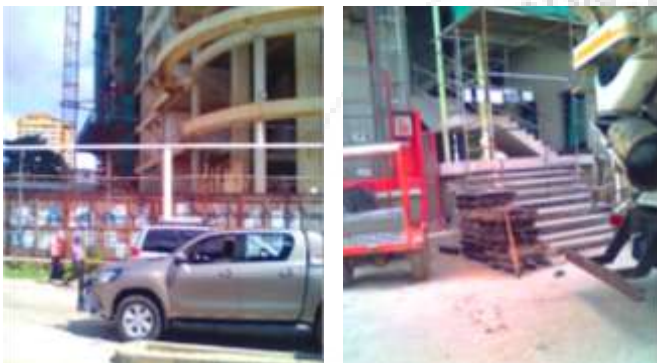
Plate 4.03: (Left) tower crane within confined site; and (Right) large concrete mixer within confined site Source: Author,(2017).
