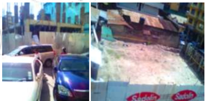
Plate 4.07: (right) confined construction sites restricted by other existing structures; and (left) outside environment of a confined building construction site, Source: Author,(2017).
