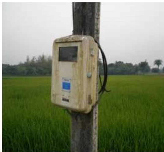
Electric Meter Box
