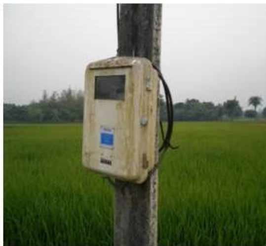
Electric Meter Box
