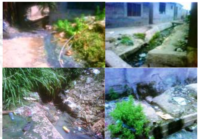
Figure 4.03: Storm water drainage systems blockage from solid waste accumulation, Source; Authors, (2017).
