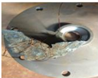
Figure 6: Corroded Zinc Anode
