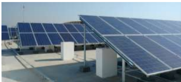
Figure 2: 100 kW p rooftop solar power plant at Poornima University
