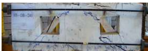
Figure 13: Crack pattern at ultimate load for beam HS-DB-240 (Group B) (diagonal splitting failure)
