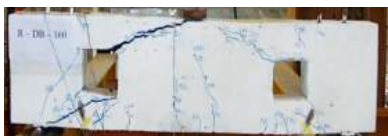
Figure 9: Crack pattern at ultimate load for beam R-DB-160 (Group A) (diagonal splitting failure)
