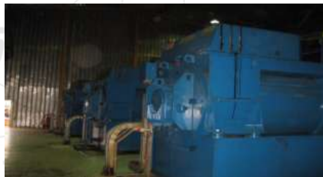
Figure 1: Engine room at OYOM-ABANG I
