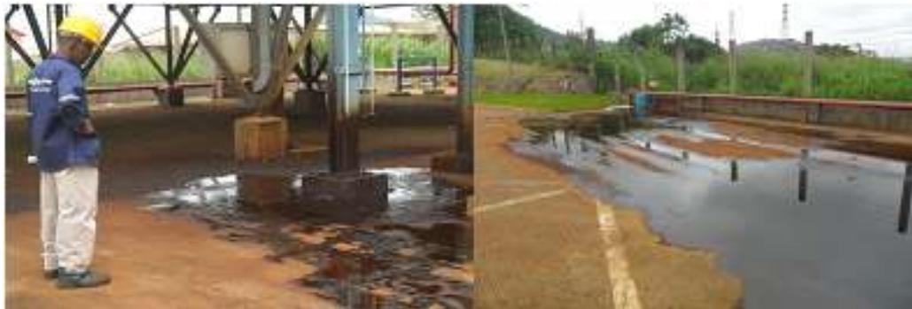
Figure 12: Dumping of products in the receiving environment due to a leak in the coolant-oil heat exchanger coming out of the bleed (TPO)
