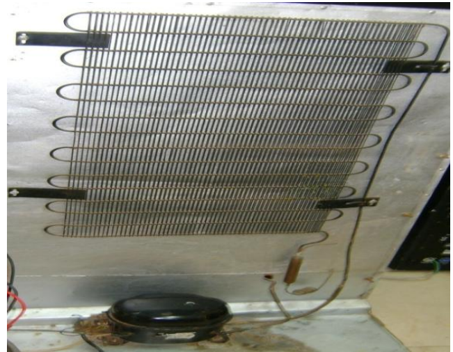
Figure 3: Shows the back of the normal refrigerator
