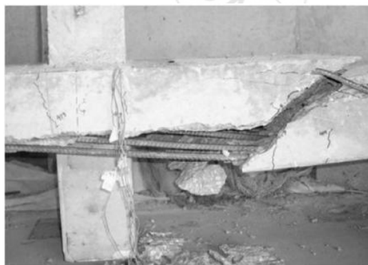
Figure 4: A photo shows beam after failure
