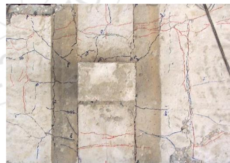
Figure 3: Cracking pattern on the top surface of beam.
