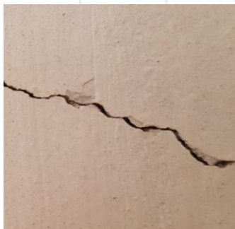
Figure 1.1: Crack on a surface wall
