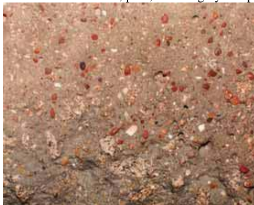
Figure 1.1: Color change in the concrete due to elevated temperature
