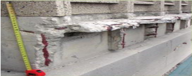
Figure 3: Spalls in concrete
