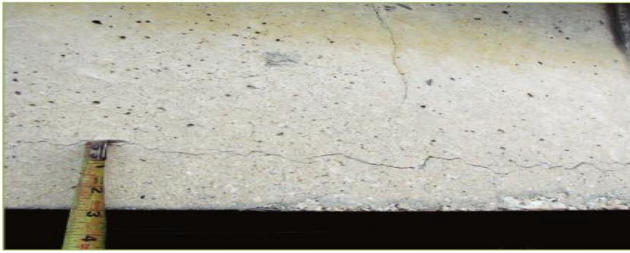
Figure 2: Cracks in Concrete
