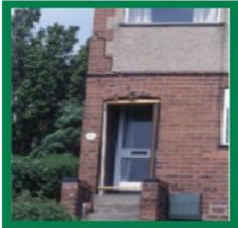
Figure 6: Differential Settlement Due to Influence of Trees
