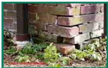
Figure 2 : Brick Foundation Damages Showing the mortar damages due to flood
