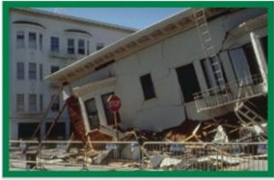
Figure 4: Damages of Building/ Foundation Due to Earthquake /Liquefaction
