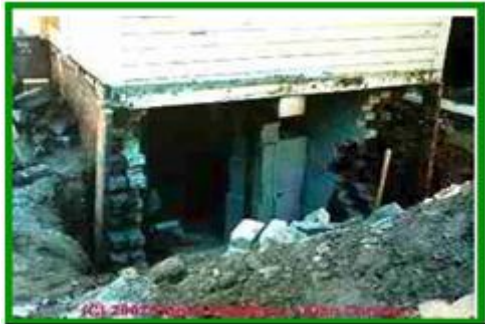
Figure 1: Damage of Brick Foundation Due to Wet Soil / Drainage Problem
