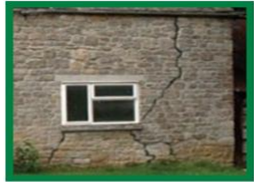
Figure 3: Development of cracks In Buildings Due to differential Settlement of Foundations
