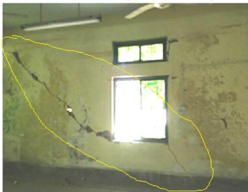
Figure 2: Long Wall of Sir Alexander Cunningham hall (political block) Width- above 2mm Type- Wide (Non-structural crack) Shape- Stair step crack Cause- settlement of foundation.
