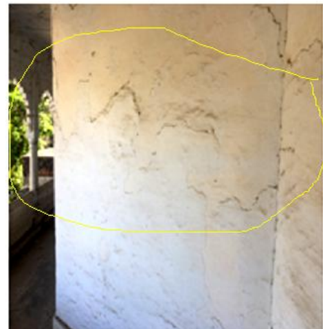
Figure 2: Wall of labour court Width- 1mm Type- Medium (Non-structural crack)
