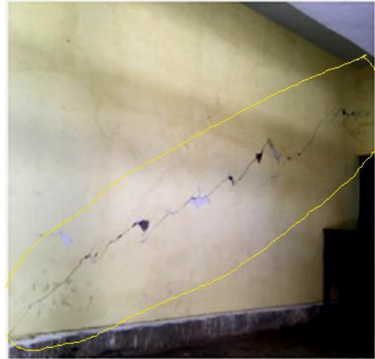
Figure 4: Wall in archaeological block Width- 1to 2 mm Type- medium, non-structural crack Shape- diagonal Cause- settlement of foundation
