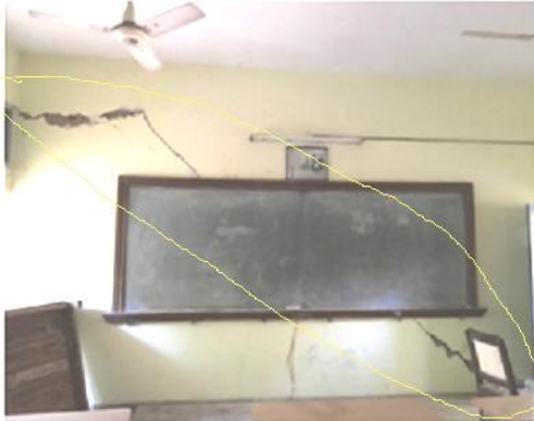
Figure 1: Short wall of classroom16 (political block) Width- above 2mm Type- Wide (Non- structure) Shape- Diagonal, Horizontal crack Cause- settlement of foundation
