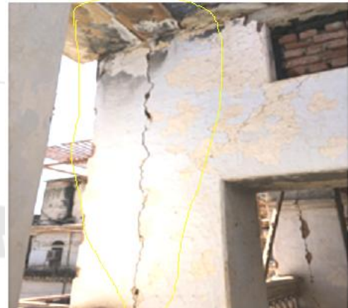
Figure 1: Column at industrial court Width- 2mm Type- Major structure Crack Shape- vertical crack Cause-thermal variation, due to joint
