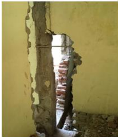
Figure 3: Rear column Type- Major Structural crack. Cause- settlement of foundation.
