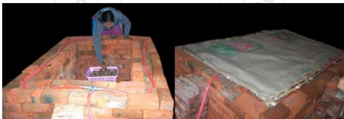
Storage area for vegetables in cool chamber Top of the cool chamber & water supply
