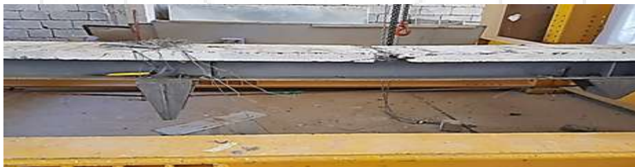
Figure 13: The Mode of Failure of the Steel Girder (GP9D-e160) G6
