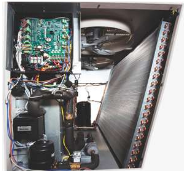
Figure 2.2: The arrangement of pumps, compressor, data cool controller
