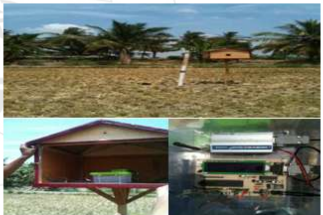
Figure 7: Sensor Equipment Water level
