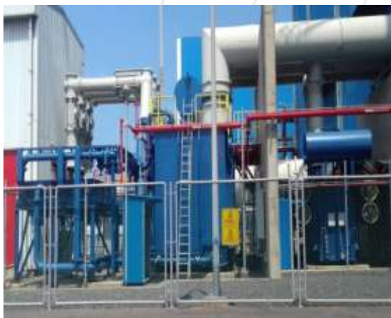
Figure 1: Power transformers of 500 kV in PT. YTL
