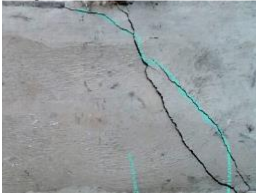
Figure 14: Crack width on beam incorporating ferrocement formwork
