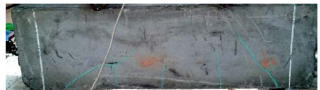
Figure 12: Crack pattern of beam with ferrocement formwork having double layers of chicken mesh
