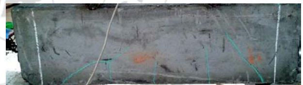
Figure 12: Crack pattern of beam with ferrocement formwork having double layers of chicken mesh
