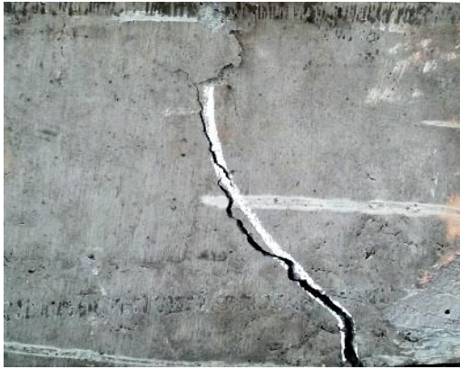
Figure 13: Crack width on control beam
