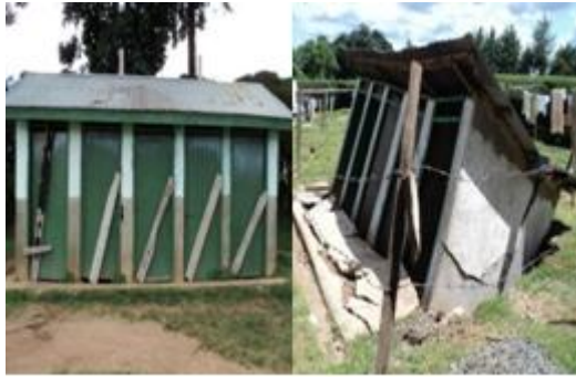
Plate 3a: Condemned & Plate 3b Collapsed pit latrine
