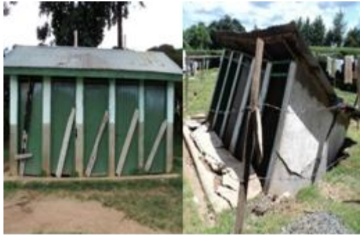
Plate 3a: Condemned & Plate 3b Collapsed pit latrine
