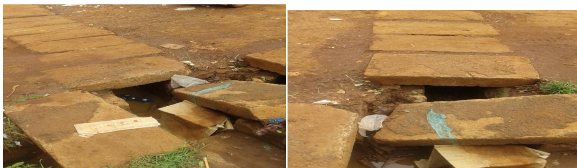
Figure 6: Poorly Covered open drains
