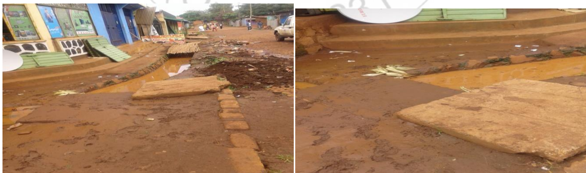
Figure 2: Rectangular Open Drains with poorly defined outlet
