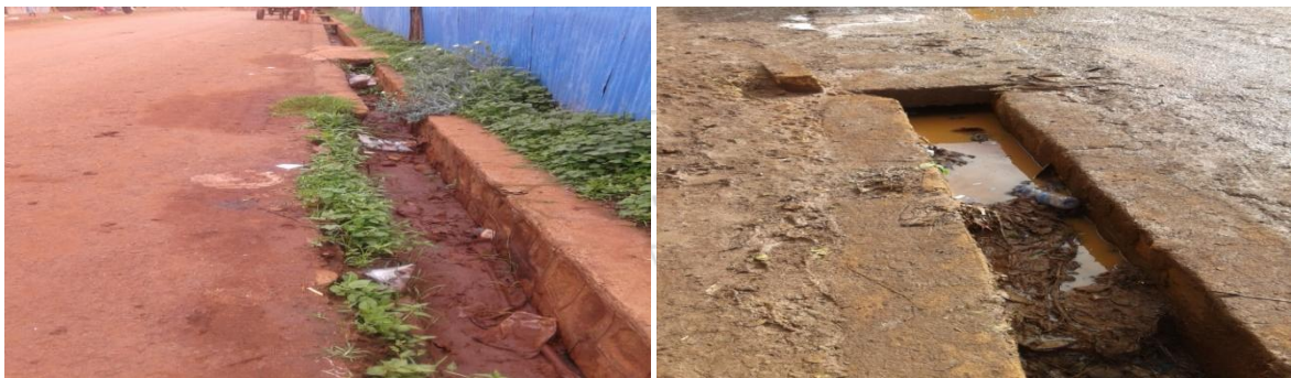
Figure 4: Failed & blocked Side drains
