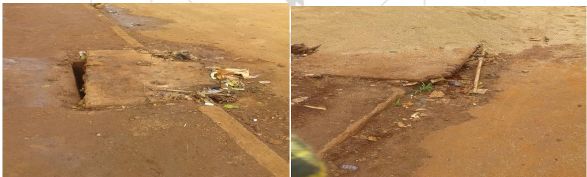
Figure 5: Poorly Executed Manholes
