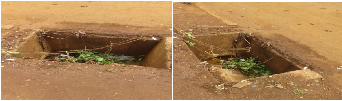
Figure 3: Manholes used as dump place
