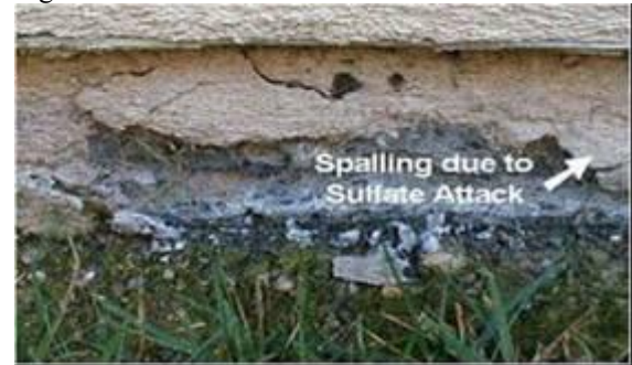
Figure 2: Spalling due to sulphate attack
