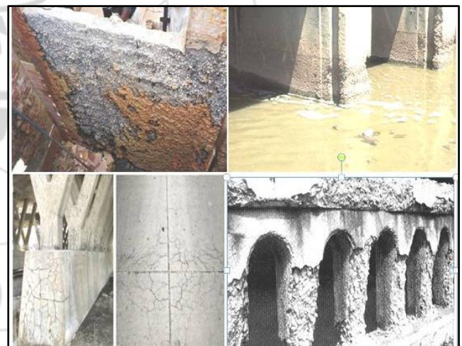
Figure 1: Deterioration of concrete structures (anticlockwise from top left) (Chemical reactions, Aggressive water attack, Freeze and thaw process and alkali silica attack)
