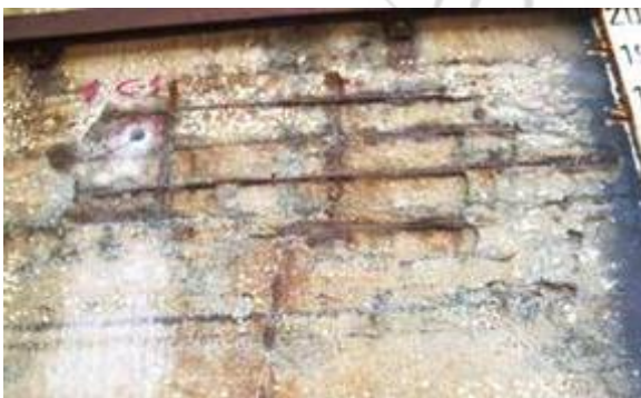
Figure 6: Corrosion of steel reinforcement due to chloride attack
