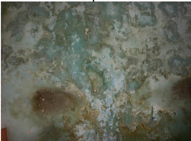
Photo-Dampness in Plaster
