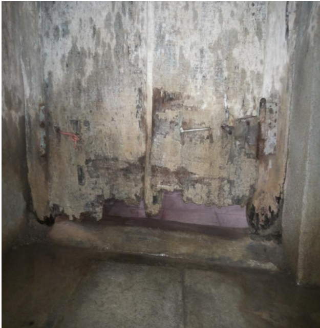
Photo- Dampness in Doors
