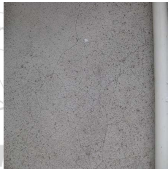
Photo- Surface Cracks on Plaster
