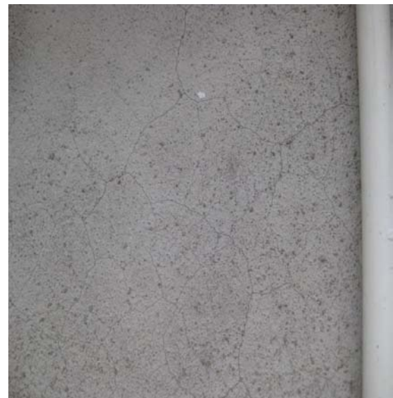
Photo- Surface Cracks on Plaster
