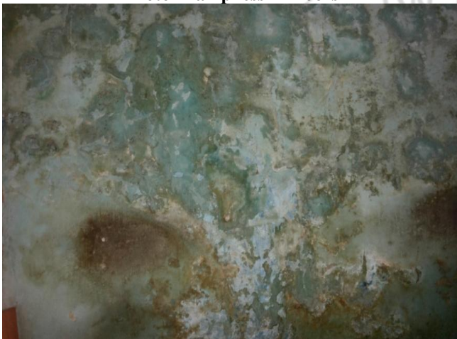
Photo-Dampness in Plaster
