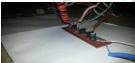
Figure 2: Power supply unit
