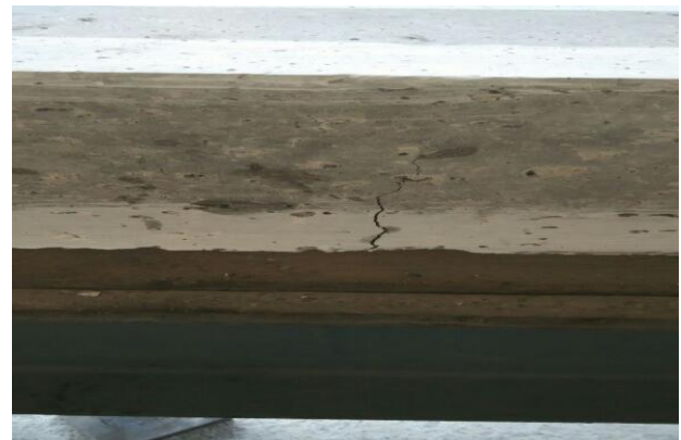
Figure 11: 15mm crack termed as first crack
