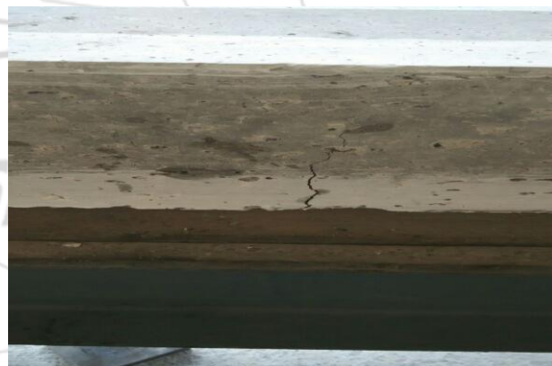
Figure 11: 15mm crack termed as first crack
