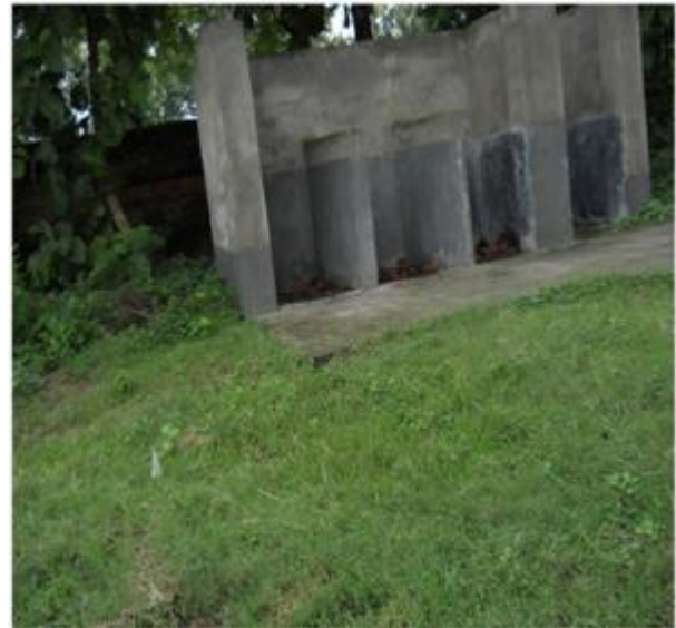
Plate 3: Poor Toilet facility in Sakti mandir harivushan das Primary School, Krishnagar
