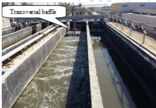
Photo 3: Transversal baffle situated ahead of end wall of the grit removal chambers at new municipal wastewater treatment plant of Kufa, Iraq.
