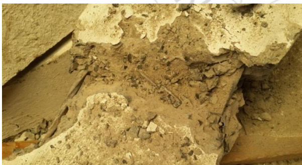
Figure 16: Snapped shear reinforcement for steel 1x6 beam
