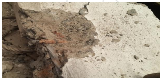
Figure 8: Unbroken shear reinforcement for L.B.1x6 beam
