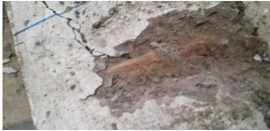
Figure 12: Unbroken shear reinforcement for L.B.2x10 beam
