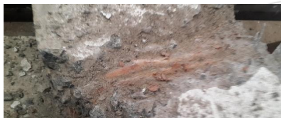
Figure 14: Unbroken shear reinforcement for L.B.2x13 beam
