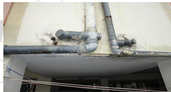
Distress Found in Sanitary System
