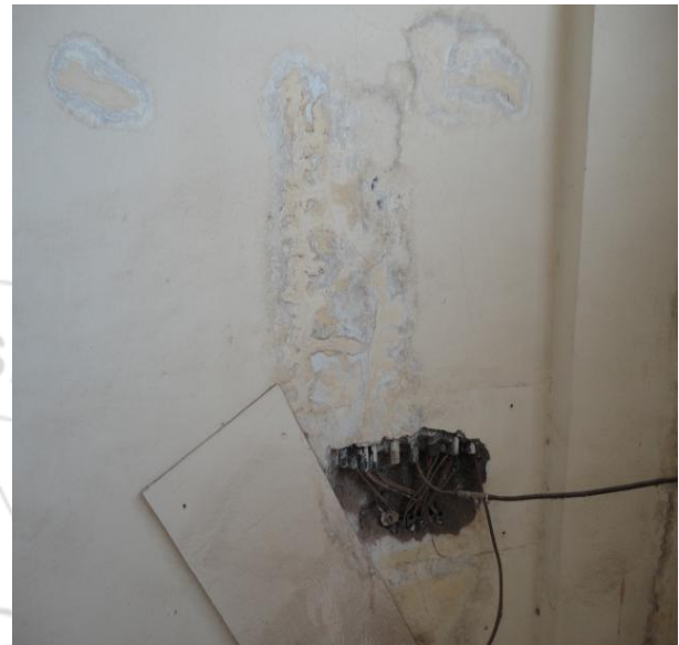
Distress Found in Switch Board
