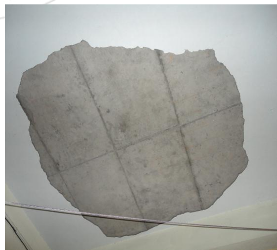
Distress Found in Roof
