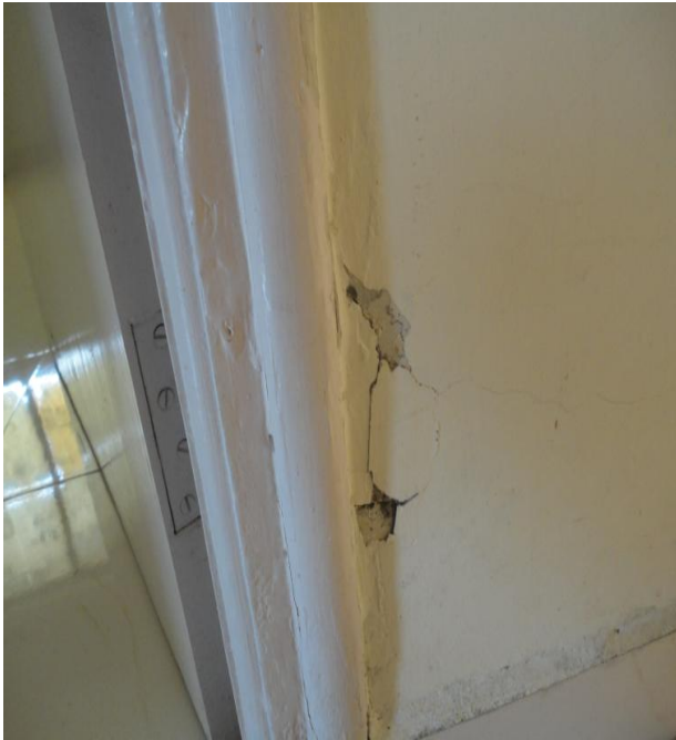
Distress Found in Wall
