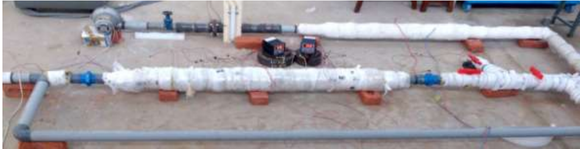
Figure 1.8: Photographic view of experimental setup (duct side)
